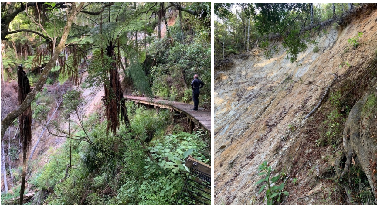
FIGURE 8: TRUE RIGHT BANK SLIP
