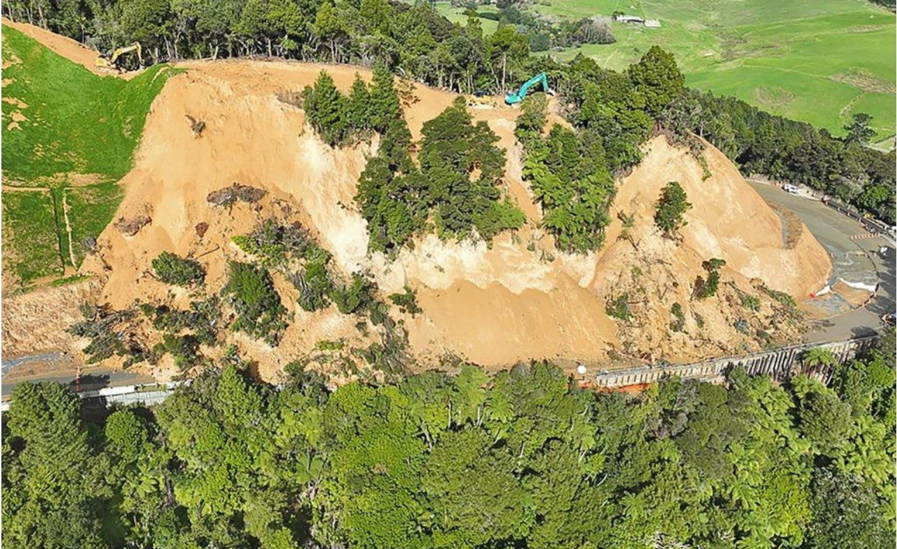
FIGURE 3: BRYNDERWYN HILLS HYDROSEEDING FAILURE
