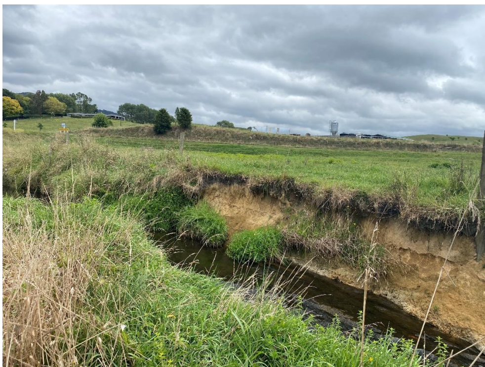
Figure 3: Stream bank erosion where flow path of Piakonui stream was altered in the past
