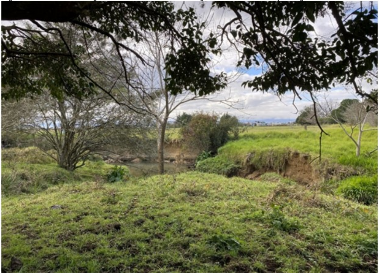
Figure 7. Bank scour and mass wasting along TRB.
