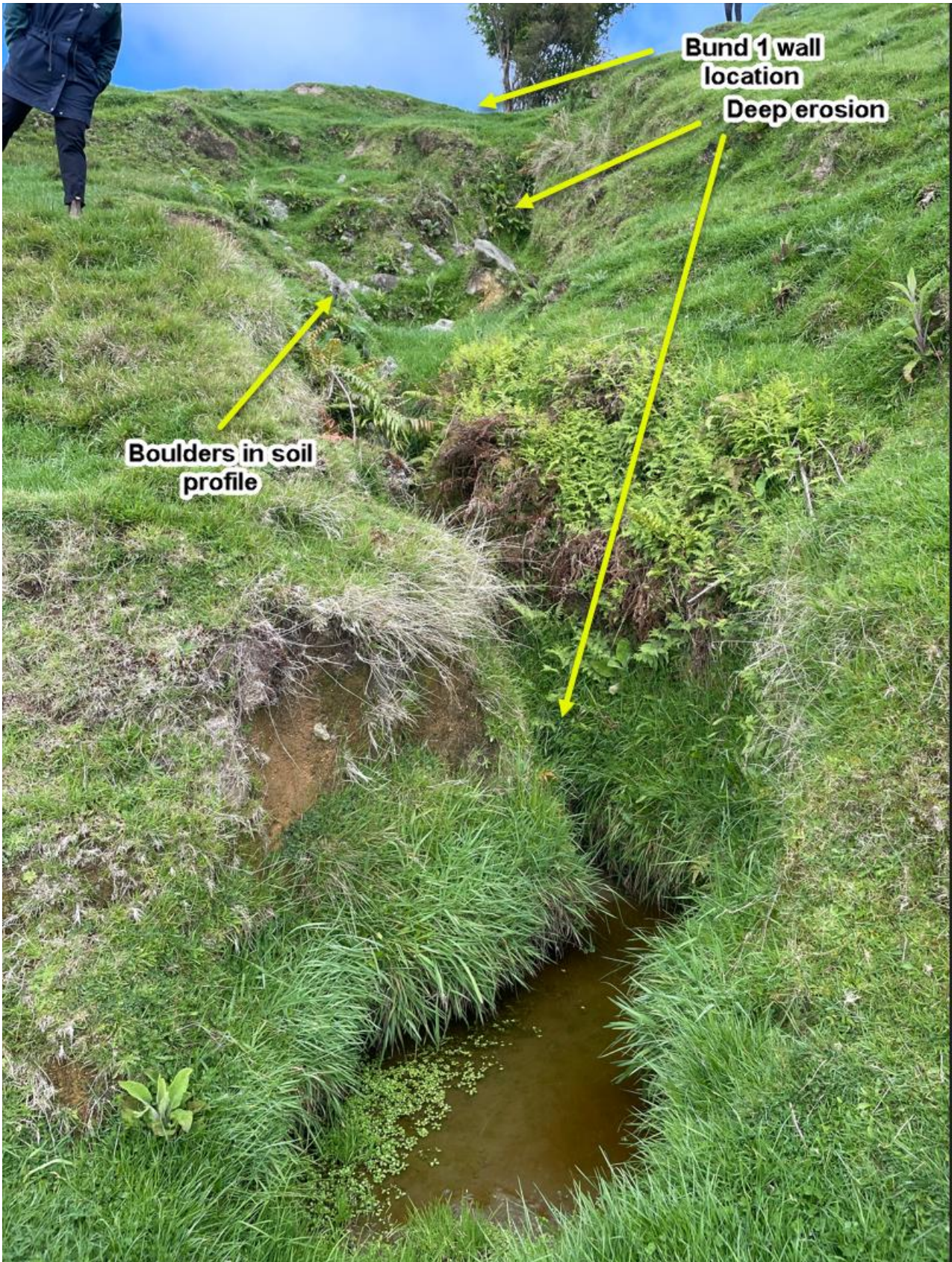
Figure B.2A View upwards from downslope of the proposed bigger bund wall. Note the steep slope, deep erosional features and large angular boulders in the soil profile.
